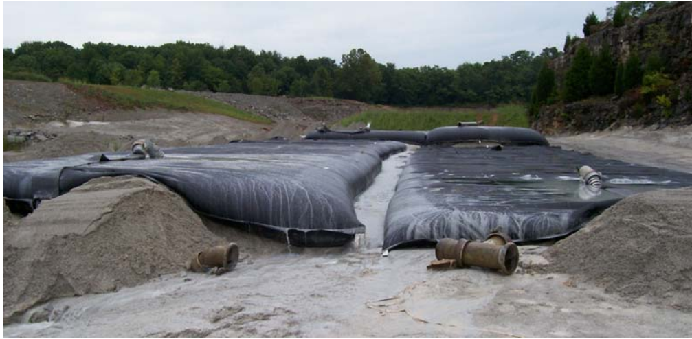
Figure 6. Solve 9350 was used to facilitate dewatering and consolidation of 850 gpm aggregate sediments in 45-ft circumference Geotubes.
