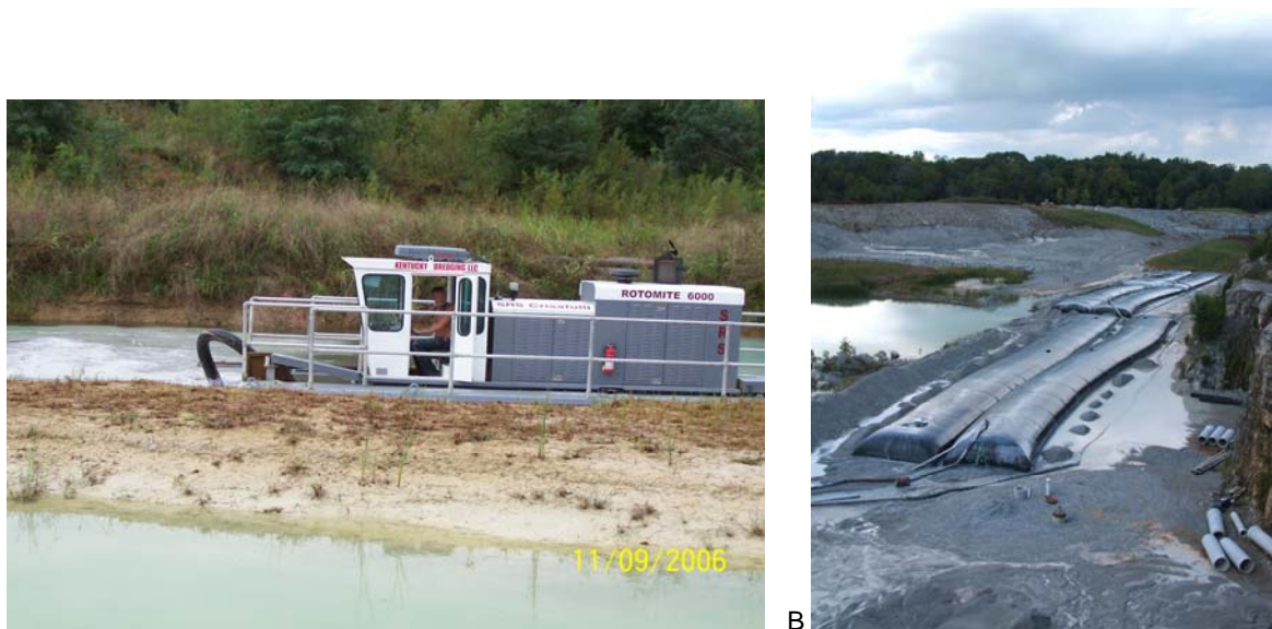
Figure 5. Retention basin sediments were dredged by Kentucky Dredge’s 8-in Crisafulli Rotomite 6000 auger dredge (A). Six hundred linear feet of Geotube consolidated to greater than 85% dry wt solids providing a permanent high-water berm (B).
