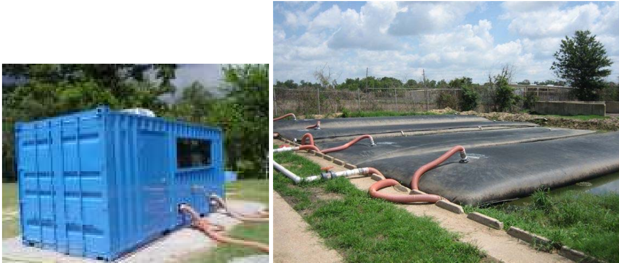
Figure 3 – Twenty eight 30-ft circumference x 50-ft long Geotube® containers were installed in existing drying beds to contain and dewater approximately four million gallons of biosolids over four months.
